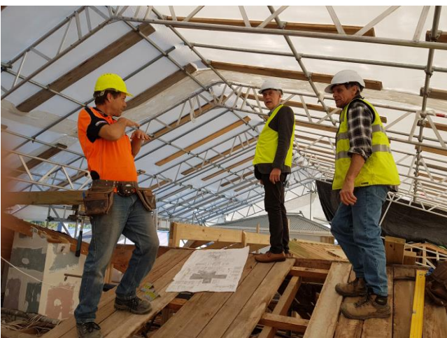
Pictured here CEO John Wigglesworth checks progress with Principal Contractor Simon Land and Project Supervisor Brian Crooks
